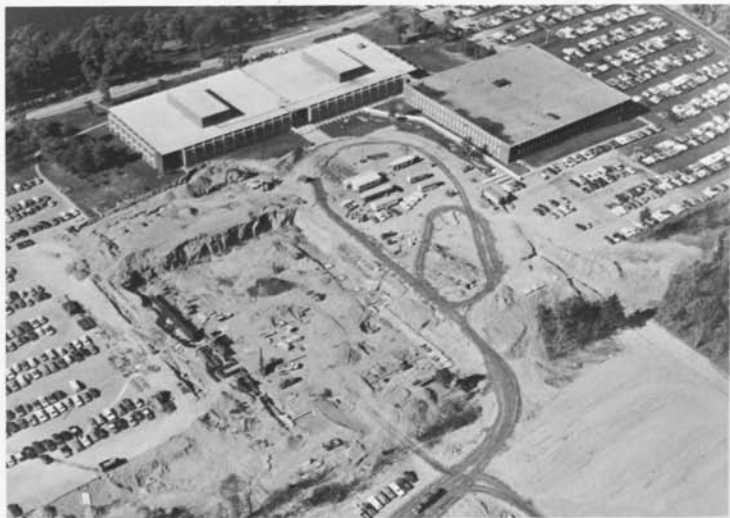
▲ Building 705 with building 706 to the north and excavation site for the new building 707 to the south.
